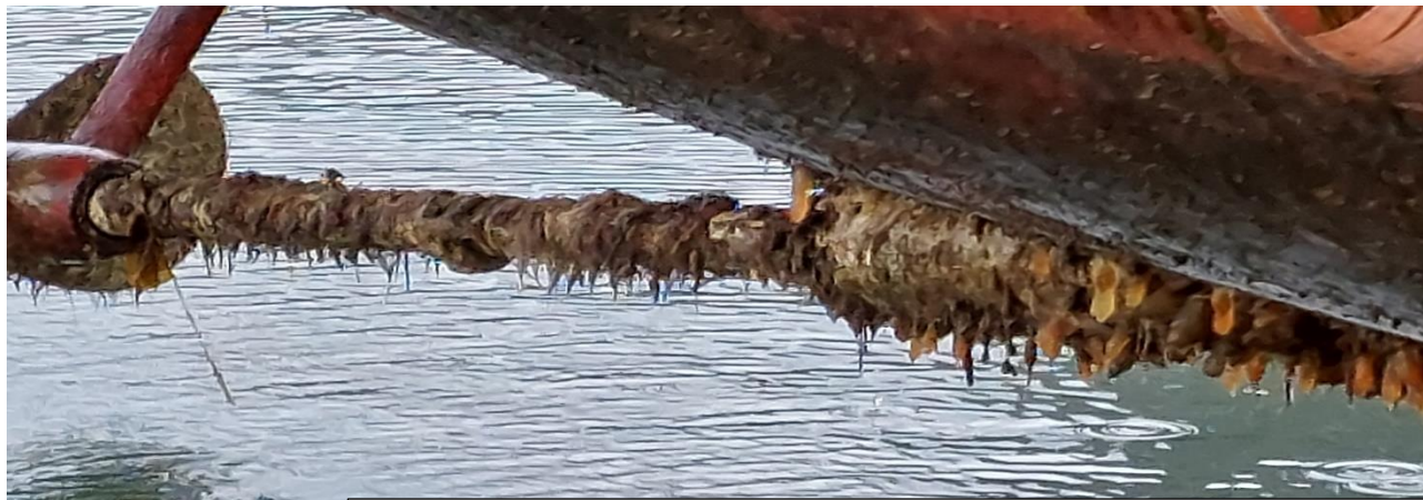
The garden like state of the shaft after lifting out by Brian M
